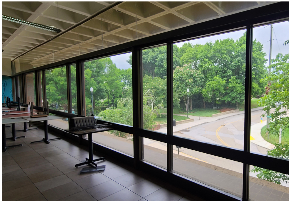
(above) View of existing exterior glass wall system at the existing Dining area.
