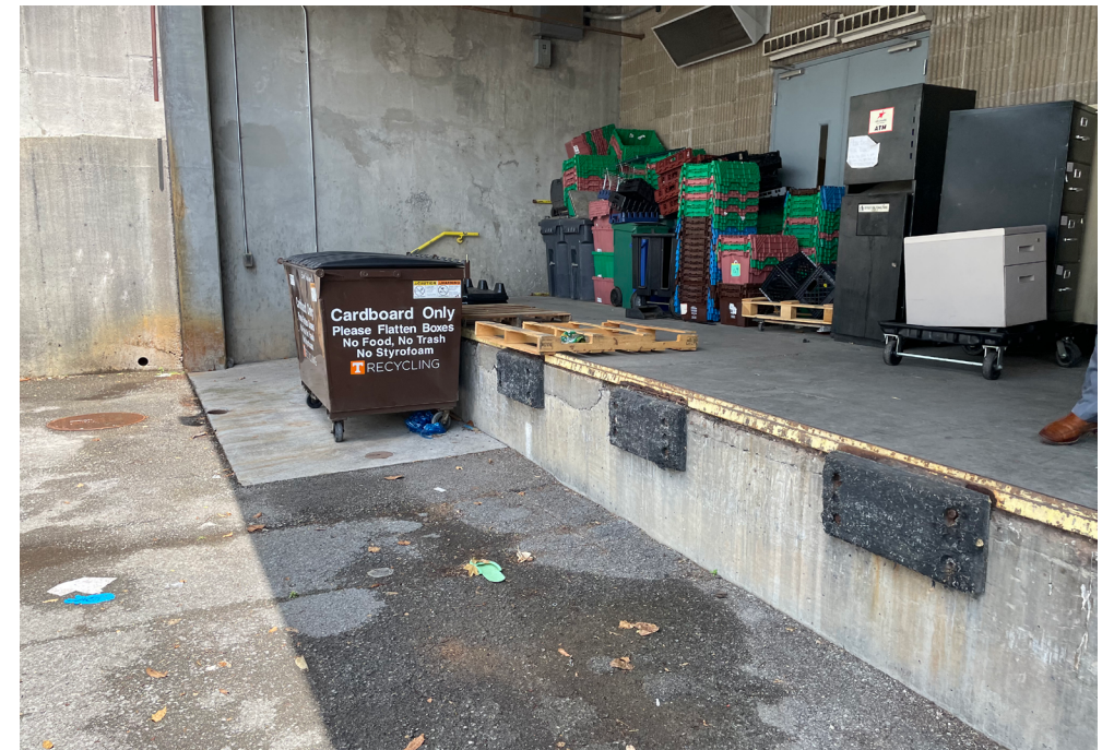
(above) Existing Loading Dock; view of proposed new ramp location for Food Service Robots.
