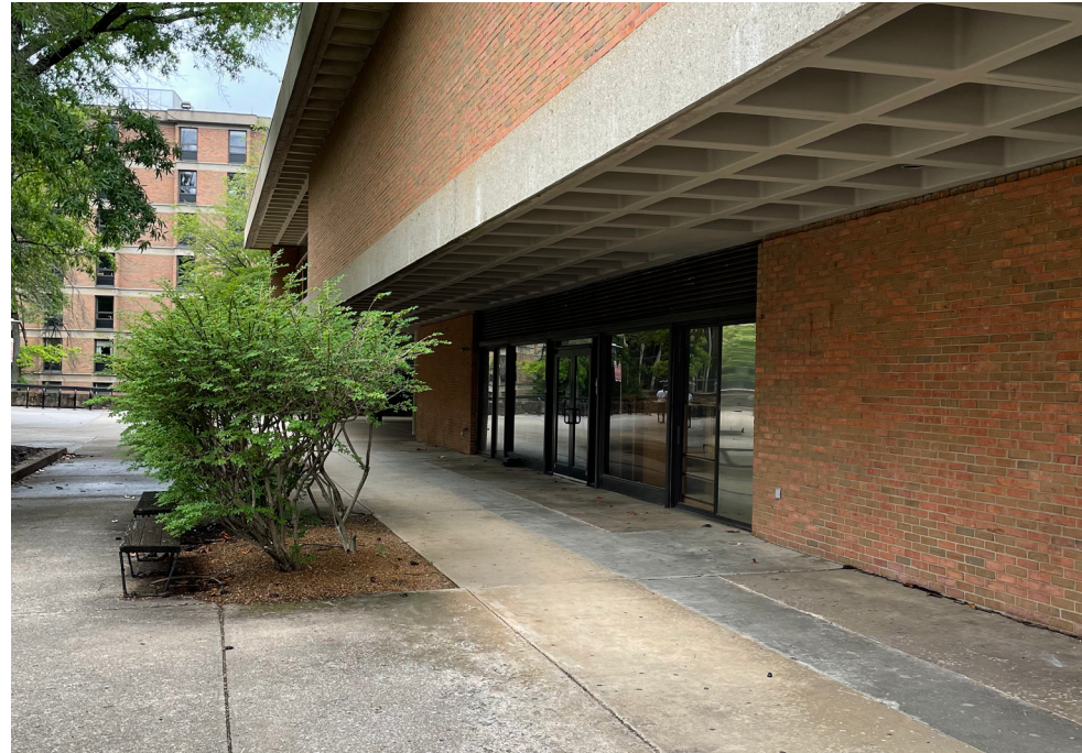
(above) Existing exterior; view of waffle slab overhangs above Ground and Second Levels.
