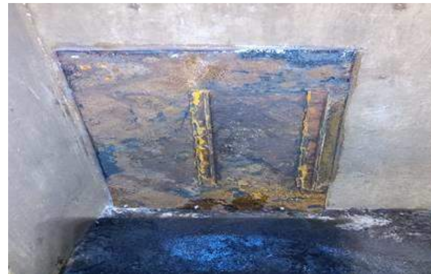
Figure 2.1.1.5 View of orifice plate relocated on the manhole wall on Oct 26, 2021.
