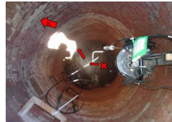
Figure 2.1.3.1. Flow meter installed at Manhole S135M222
