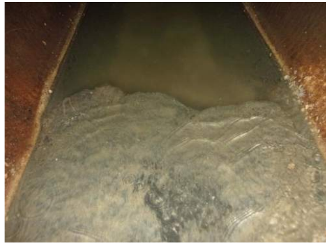
Figure 2.1.2.1. Concrete slurry on incoming 36-inch pipe to manhole S135M904
