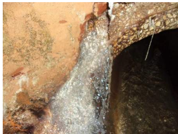
Figure 2.1.2.2. Significant I/I observed on 42-inch outgoing pipe from manhole S135M904
